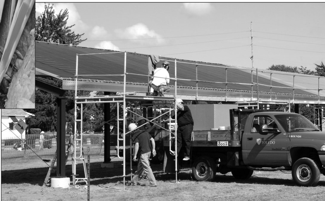
Workers installed a solar array in September on the Scott Park Campus of Energy and Innovation.
