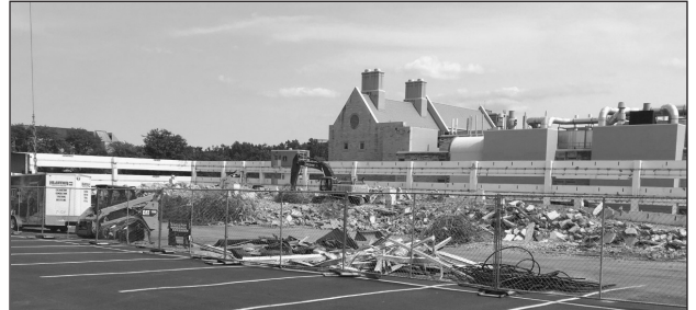
The east and west parking ramps, built in 1976, were recently demolished due to safety concerns.
